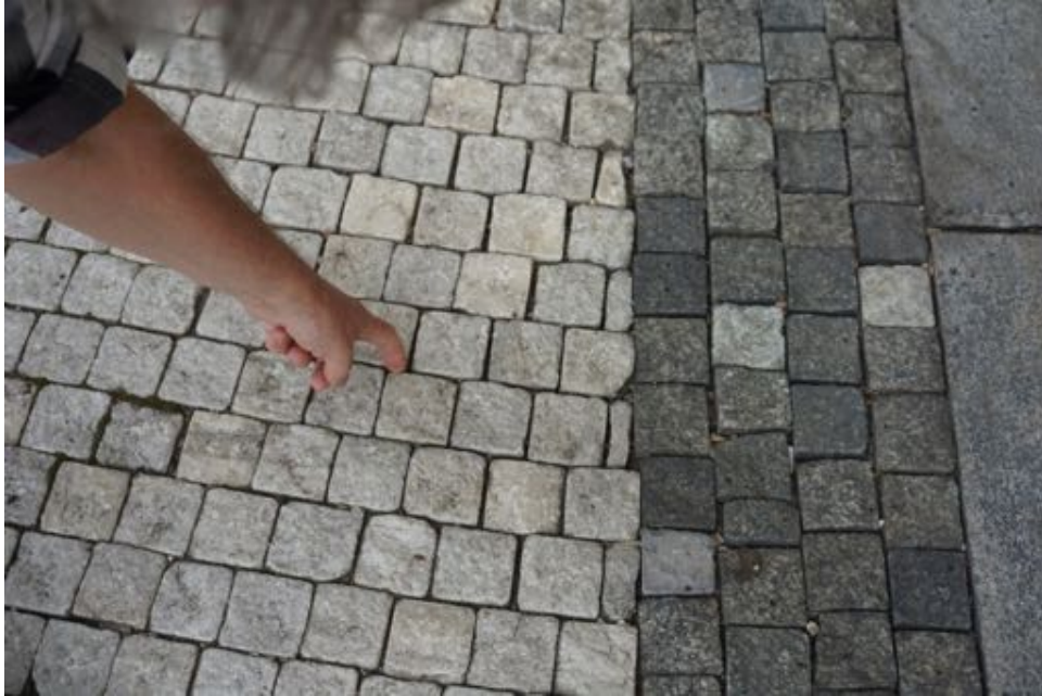
Fig. 13: Kovanda points at the gaps between the cobblestones
